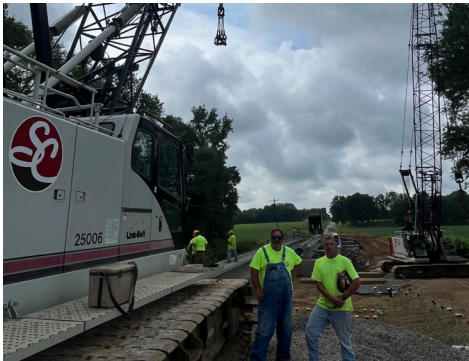
DS5 Jim Smith Contracting working on a Bridge replacement with Dan Lummus (L), Robert Cook (R)
