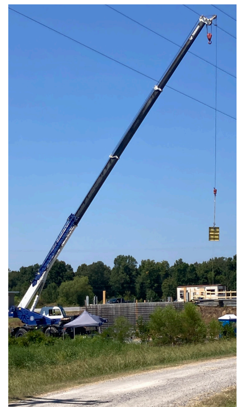
DS5 Zack Hurt working for Travis Construction at the Calvert City Water Treatment Plant
