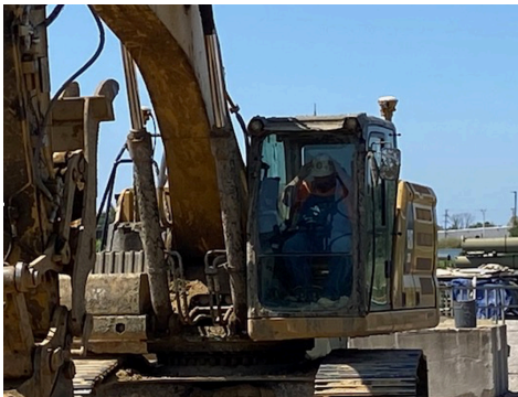
DS1 Eddie Fulkerson working for Hazex Construction Co. at Pittsburgh Tank and Tower
