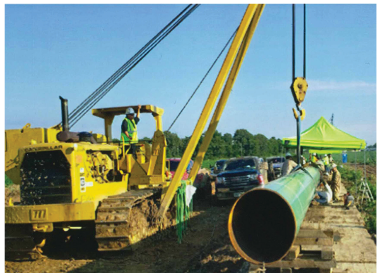
United Piping Inc. performing work on the ONEOK Kentucky Pipe Replacement project in Simpson County, KY
