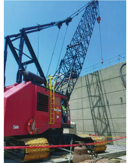
(ABOVE): C.J. Mahan on the Newburgh Lock repairs in Warrick County, Indiana (LEFT): R&R Crane Service at the Culley Station pipe replacement project in Warrick County, Indiana
