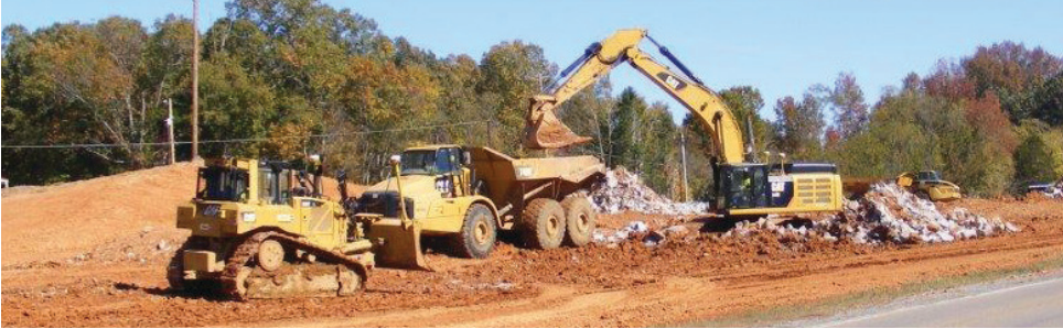
Jim Smith Contracting on the Highway 68/80 widening project in Trigg County, Kentucky
