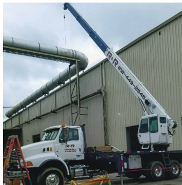
W.B. Koester performing work at the Post House project in downtown Evansville, Indiana
