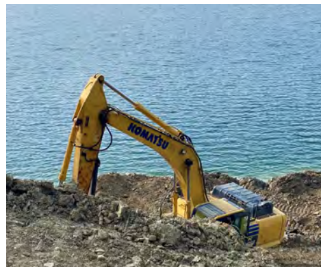
DS 6 Excavator Operator Donald Nunley working for C.J. Mahan at Cave Run Lake.
