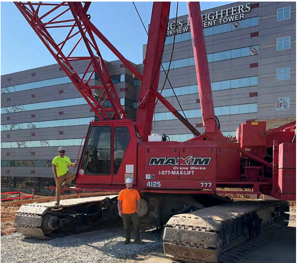
777 Crawler Crane Operator Daryl Wells with Apprentice Oiler Casey Shannon works for Maxim Crane at KDMC
