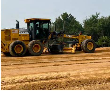
DS 2 Jeff Seifrig working for Lutgring Bros. at Spencer County Building Pad.
