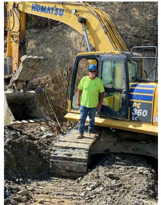
Excavator Operator Donald Nunley works for C.J. Mahan on the Cave Run Lake Raw Water Intake Project
