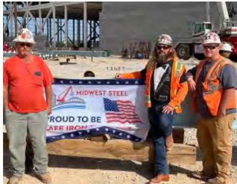
DS 1 Nathan Parrish, Josh Moss and Donald Durard working for Midwest Steet on the new battery plant in Bowling Green.
