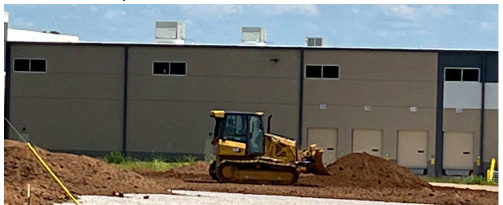
DS1 Zack Winkler working for Independence Excavating on the GM warehouse in Bowling Green.
