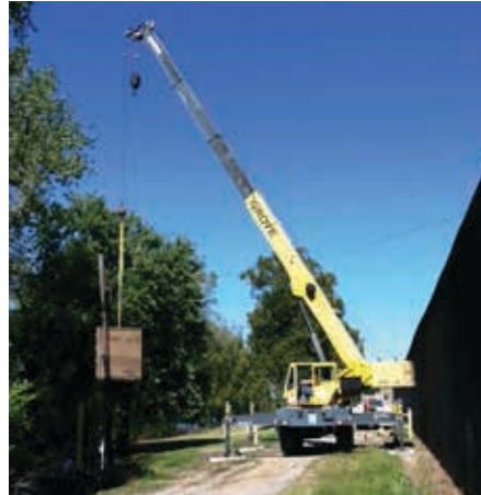
Andy Selzer, removing an old flood gate for Deig Bros. in Perry County, Indiana
