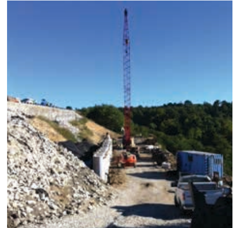
Force Construction at the State Road 237 Slide Project in Tell City, Indiana
