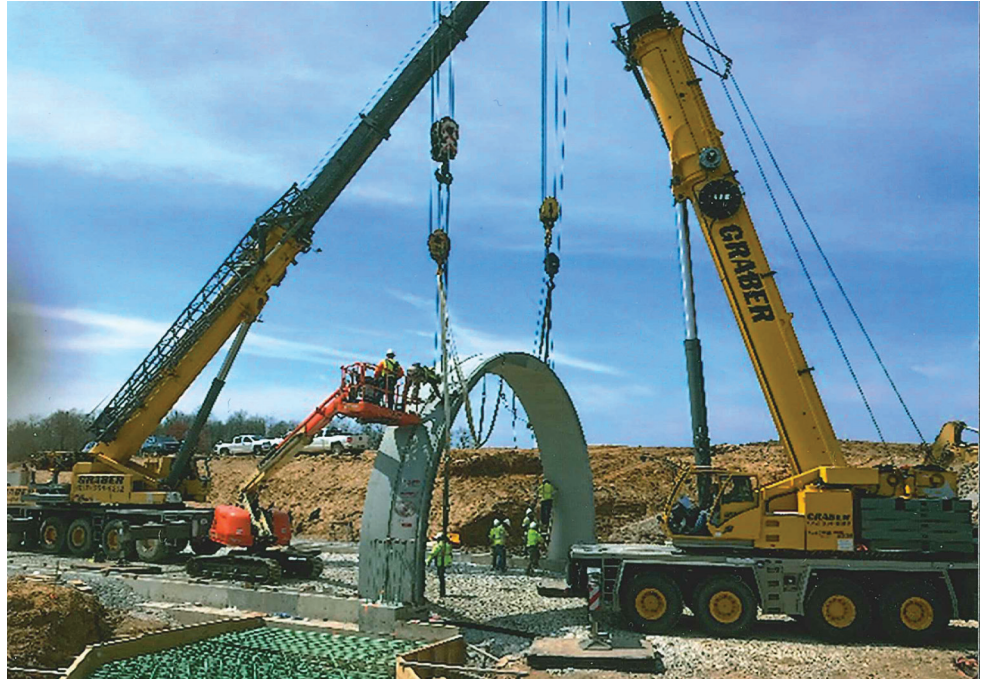
General Contractor W.B. Koester and Sub-Contractor Graber Crane on the Huntingburg Airport tunnel project and improvement project in Dubois County, IN
