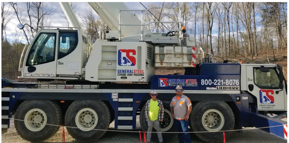
DS 4 Garrett Wells, left, oiling for Ben Watkins, right, working for General Steel in Montgomery County, Ky.
