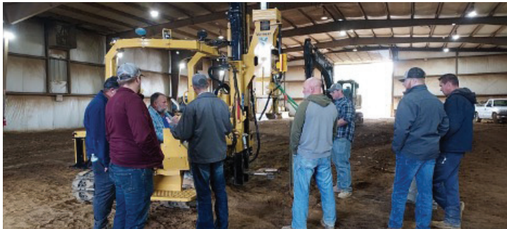
PD10 Training on Pile Driving at the Boston Training Site in preparation for possible up and coming solar field work in our jurisdiction.
