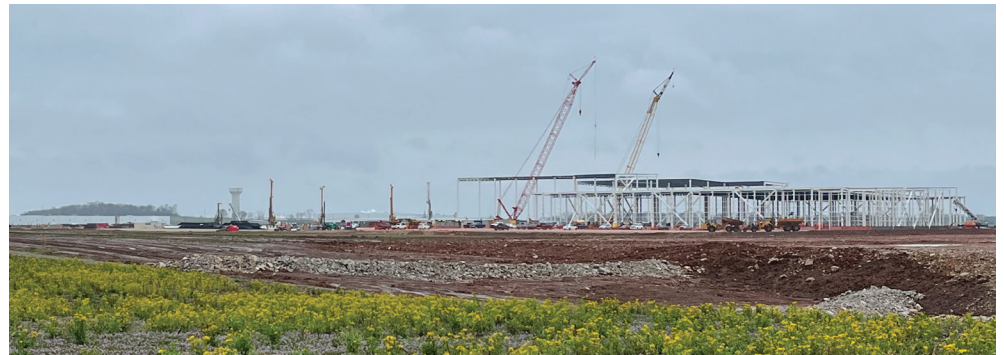
Berkel & Company and Midwest Steel at Envision Battery Plant in Bowling Green, Ky.
