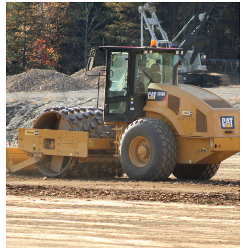
JATC-Boston Joshua Moss compacting material back into ditches after an excavation class with the Sheep Foot Roller.
