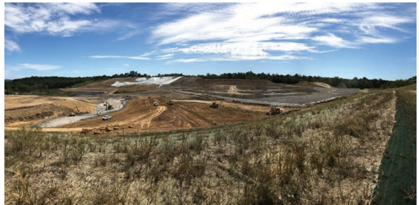
Hazex Construction on the Real Alloy Landfill Cell A & B in Butler County, KY.
