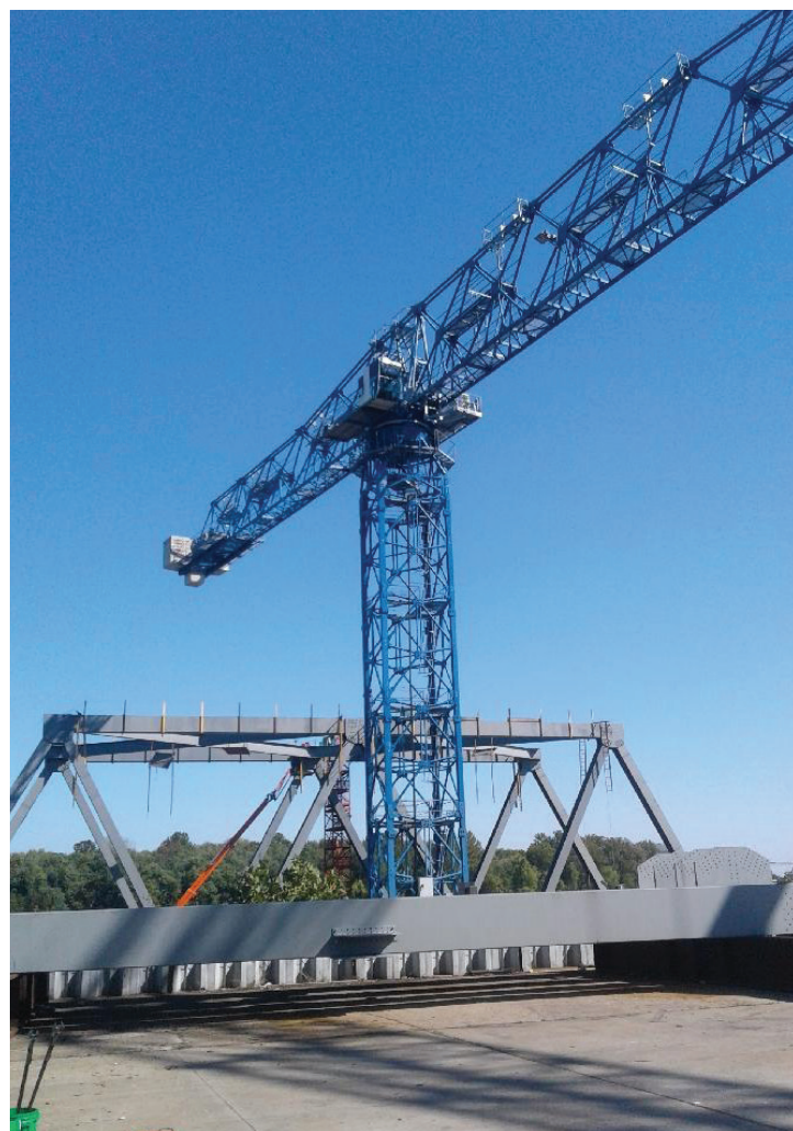
The Superstructure of the Smithland Bridge being put together at Paducah by American Bridge
