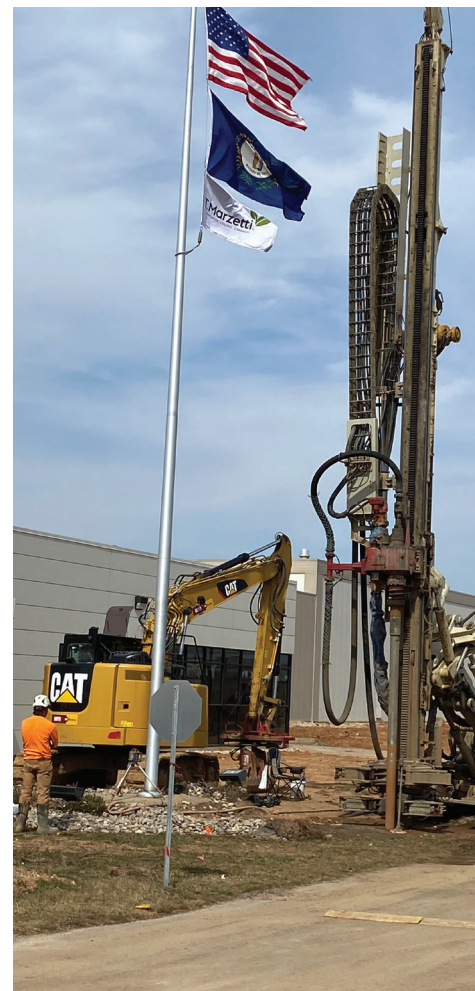
T Marzetti expansion in Horse Cave, KY. Work being done by Keller North American
